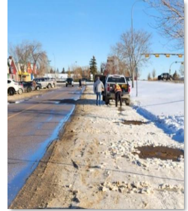
Sensor installation in on-street parking spaces
